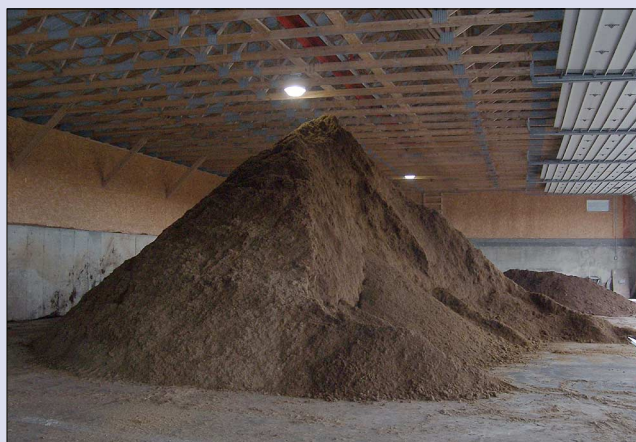
An anaerobic digester at the Blue Spruce Farm in Bridgport, Vt., turns manure into odorless solids that can be used for cow bedding, as well as methane that can be burned to generate electricity.
