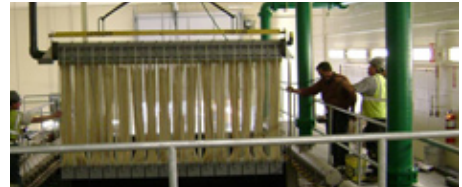
Sewage Treatment Plants
