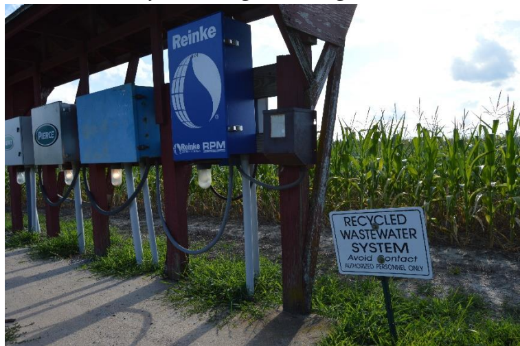
The wastewater pumping system outside at the Mountaire slaughterhouse in Millsboro, Delaware, next to the corn fields, where the waste is sprayed
